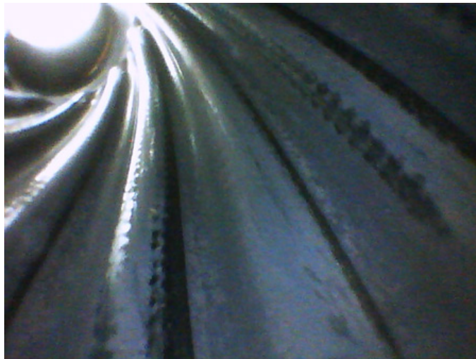
Figure 4 - Post-run borescope of stator
